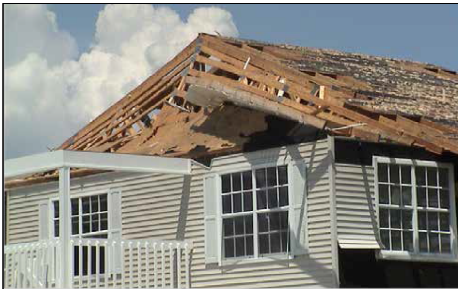
Figure A-7. The most common gable end failure is one where the wall loses support along its top edge because sheathing is blown off. The wall may fold outward (see cover picture) or be blown inward.
