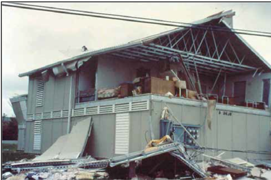
Figure A-9. The more usual result of wall connection failures is a missing gable end wall and the wall below.
