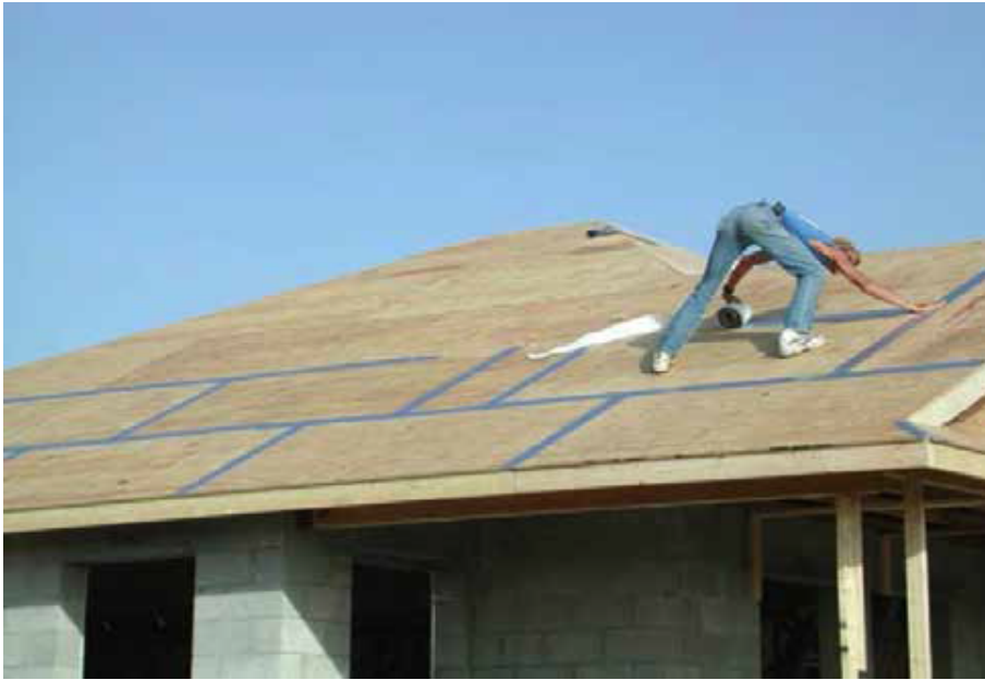
Figure 6. Installing a Sealed Roof Deck System; Taping the Seams of Roof Sheathing
