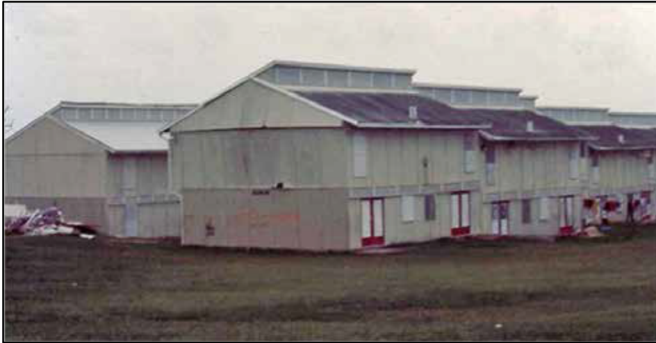
Figure A-8. The second most common type of gable end failure is at the connection between the rectangular and triangular walls. Here, the failure is just starting.
